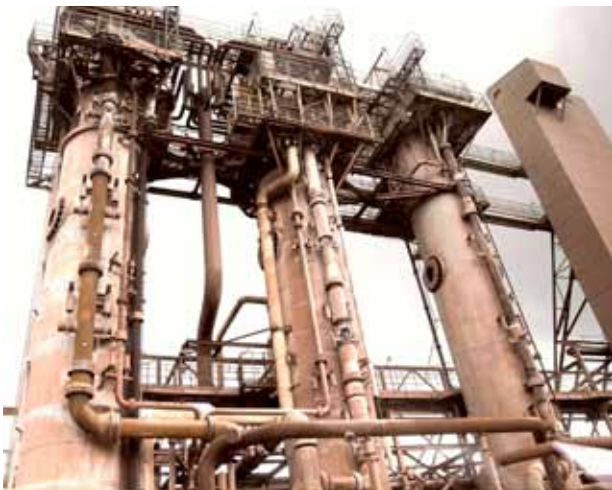
One of the digesters
