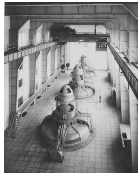
A photograph taken immediately after construction in December 1929, showing the first three turbines, the fourth was yet to be installed. Photograph: courtesy of ESB Archives
