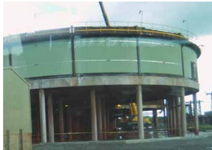
Slurry containing the red mud is pumped into one of these wide flat tanks, in which the mud gradually drops out forming a pumpable sludge
