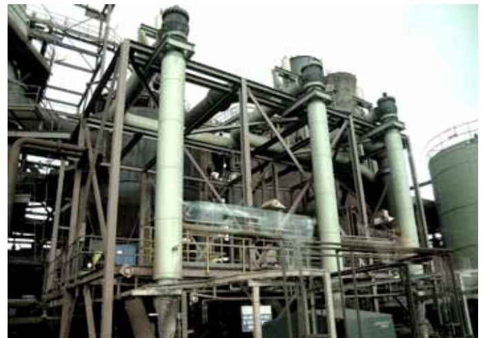
The "columns" are pipes leading from positive displacement pumps through to the final cooling stage
