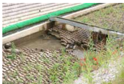
Flood damage to the Lock overflow channel by the input weir for the turbine.
