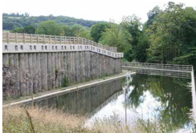
The new channel through the rubbish tip beside the railway viaduct on the right. This channel takes a very sharp turn after passing beneath the viaduct.
