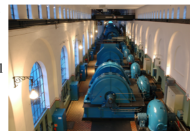
The hydropowerstation Tyssø 1, the main site and the Tyssø 1, turbine hall.
