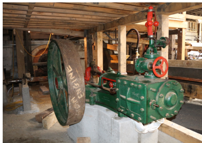
Above: The Cornish Engine House Waihi showing steel sliders on which it was moved Below: The Tangye engine at Thames gold Battery Mill
