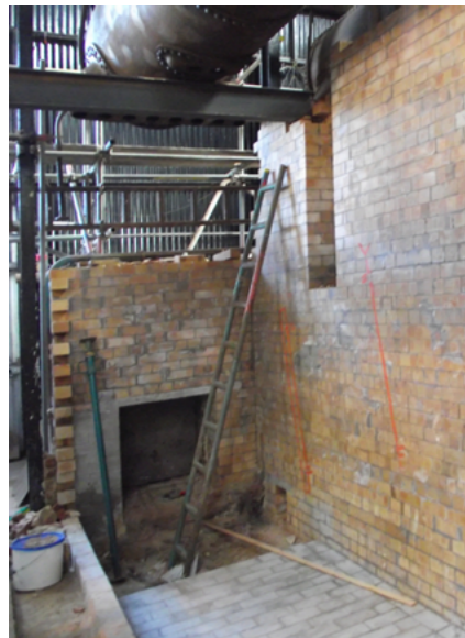
The brickwork for the 1903 boiler is complete and the figure shows the completed firebrick wall between the two boilers. The 1906 boiler is ready to be re-tubed. Image: Martin Gregory
