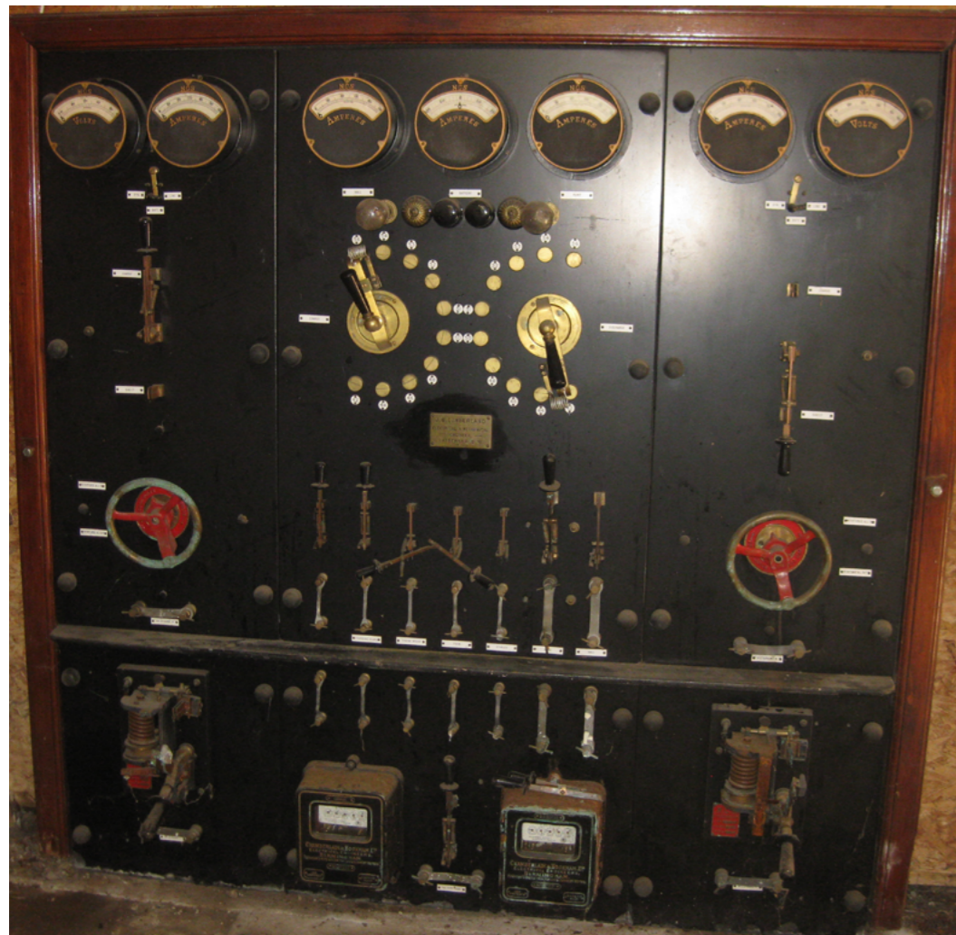
The historic switchboard before removal from Bourton Hall
