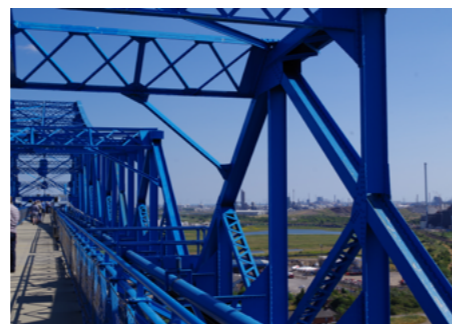
Light carbon fibre boards allow visitors to walk from one side of the Tees to the other across the high-level gantry of the Transporter Bridge. (image: Jonathan Ayles)
