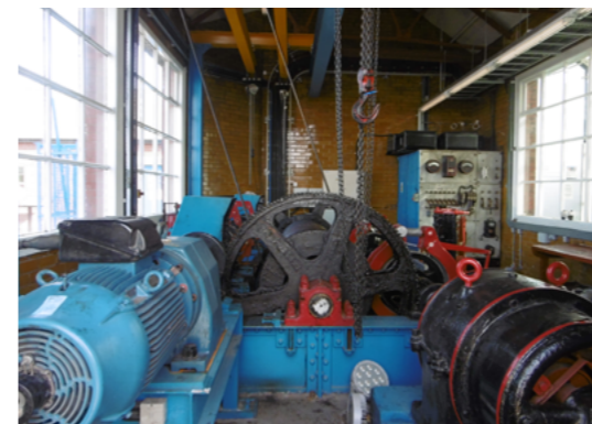
The bridge has been fitted with new AC motors, but all the original DC drive equipment has been preserved including the motors and bus bars. The machinery can be readily seen in action from a viewing booth at the back of the winding house.
