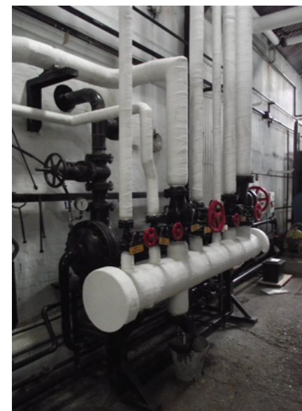
The new low-level control manifold for the boiler. Image: Martin Gregory
