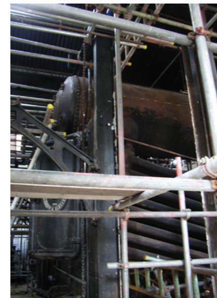
The 1916 boiler naked of brickwork and stabilised with scaffolding. Image: Martin Gregory
