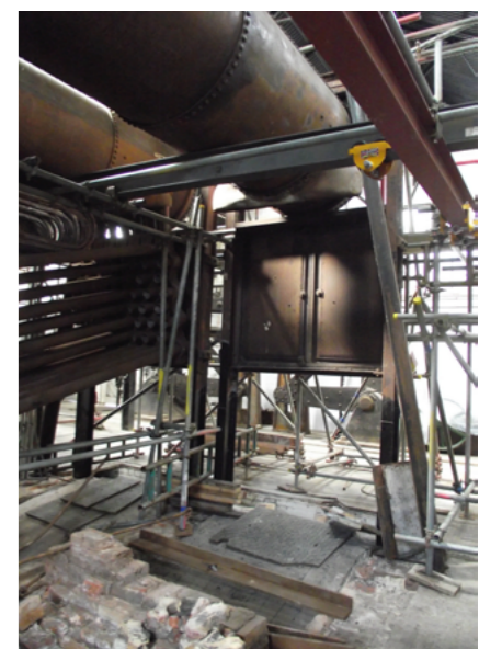
The 1903 boiler (left) still has tubes but the 1906 boiler (right) has been stripped back to the steam drum hanging from its portal frame. Image: Martin Gregory
