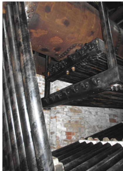
New tubes, including the superheater, have been fitted and the boiler is ready for its hydraulic test. Image: Martin Gregory
