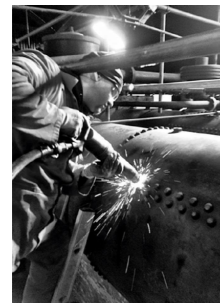
Replacing a suspect rivet on the steam drum Image: H. A. McEwen (Boiler Repairs) Ltd.
