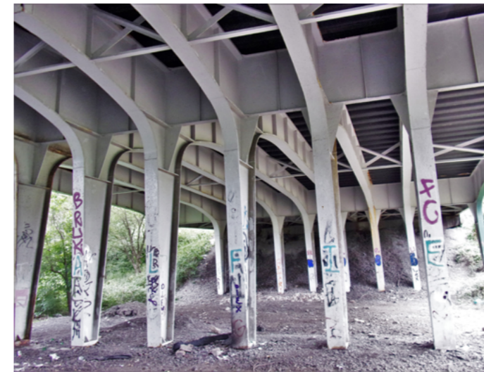
Arrangement of the columns and deck beams. Apart from the inevitable graffiti, the bridge seems to be in very good condition. Image: Fred Starr
