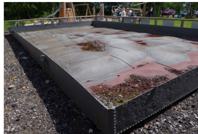
Brine tanks never stay level
